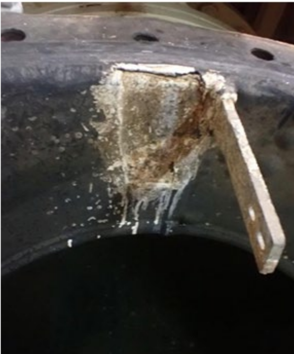
Figure: Defect area after rubber liner removal showing underlying corrosion
