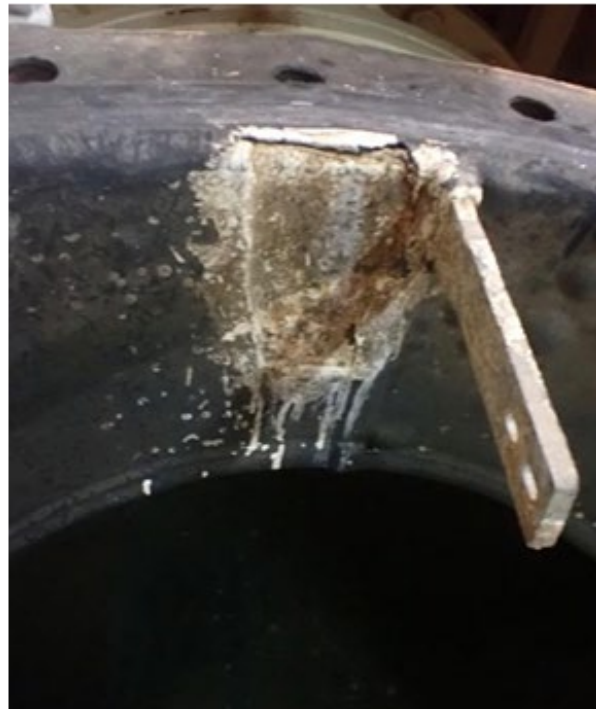
Figure: Defect area after rubber liner removal showing underlying corrosion
