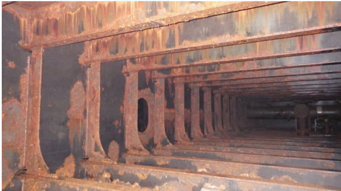
Example corroded ballast tank
