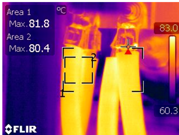
Figure 10 Cables at Position C from Window Position 1
