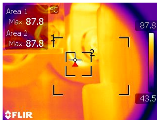
Figure 19 Bolts at Position A and Boot at Position B
