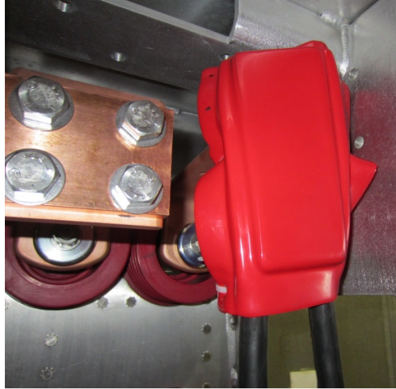
Figure 31 Rubber Boot Repositioned over Upper Phase C Connections
