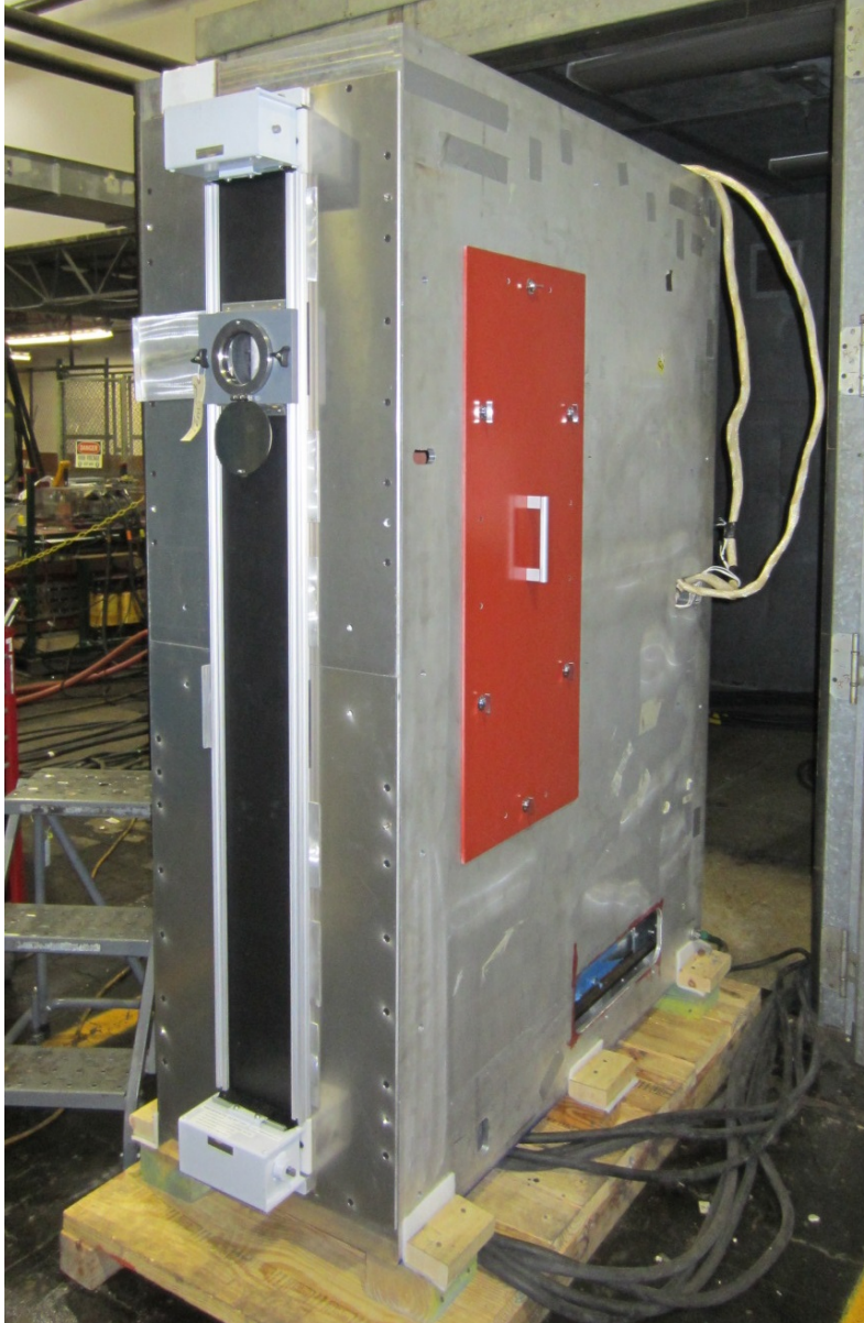
Figure 1 DRS Test Cabinet - Rear View
