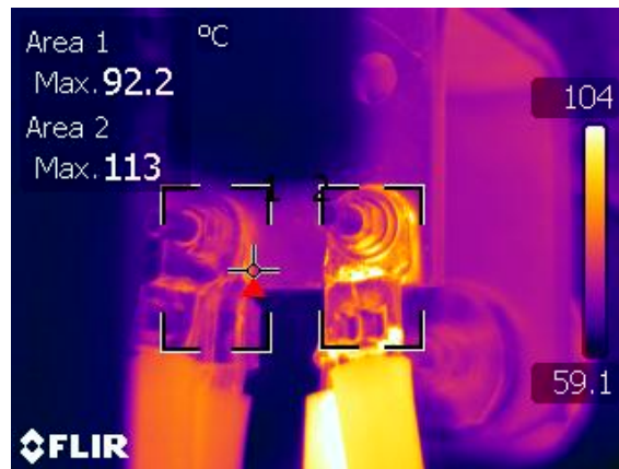
Figure 23 Fault Condition at Position C Seen From Window Position 1
