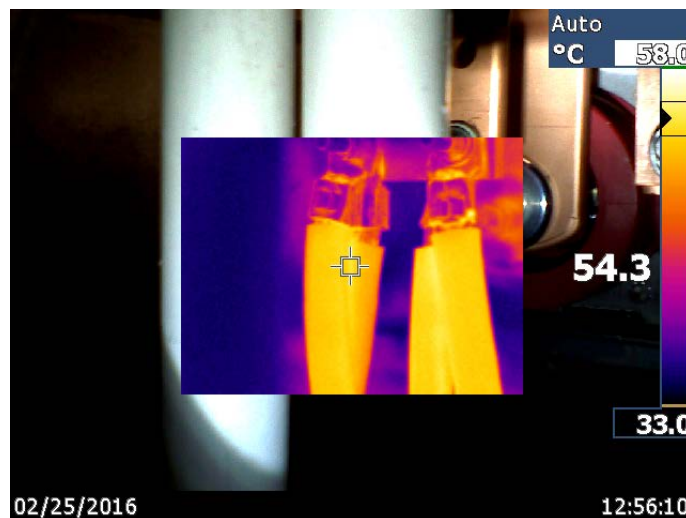
Figure 48 Fluke Camera Image of Cables at Position C, No Window
