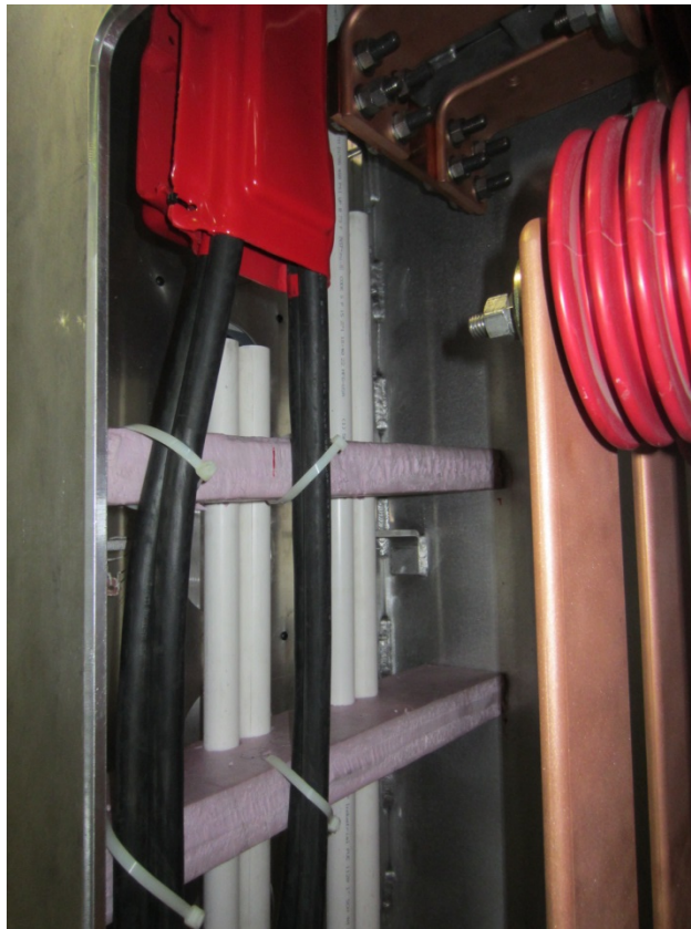
Figure 17 View of Rubber Dust Boot from Cabinet Side Opening
