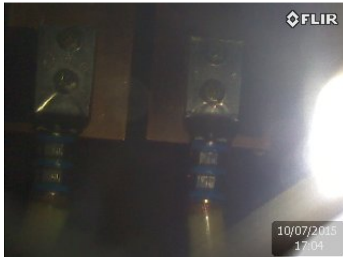
Figure 30 Digital Image through IRISS Window, Lamp On
