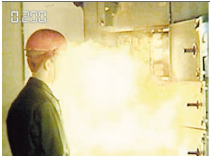
Internal core temperature may reach 20,000 °C, posing a serious threat to personnel and the switchgear assembly [Image from the ABB Review]
