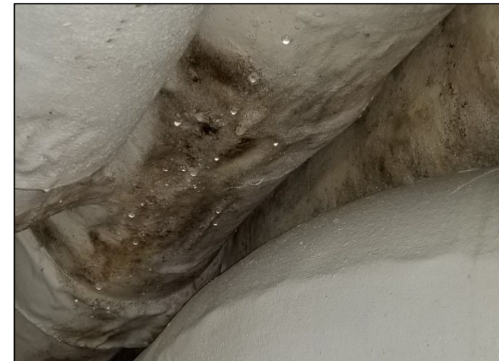
Condensation with mold growth
