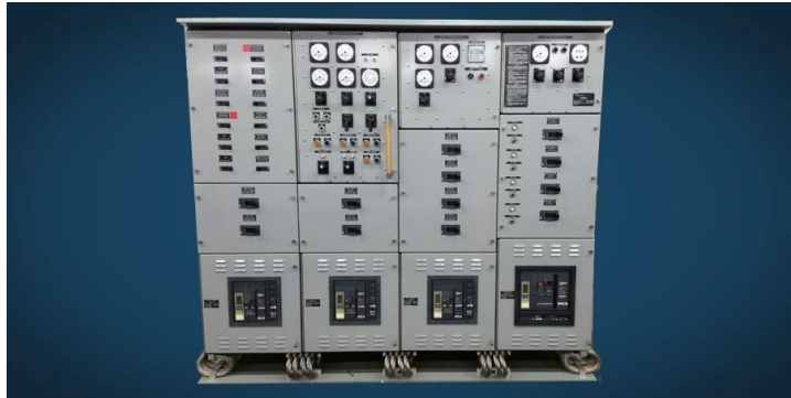
Main Distribution Switchboard
