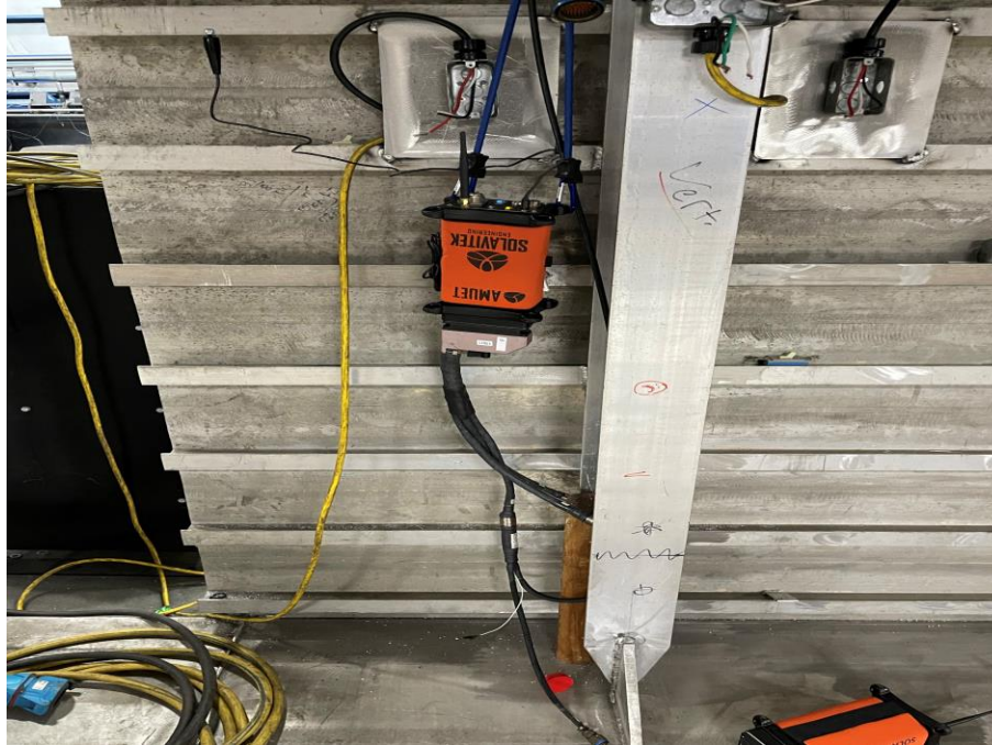
Figure 8. The AMUET tester is connected to one side of a cable to support conductor termination by the user using the smart lenses at the other end of the electrical cable. Once completed, a second identical tester will be used to complete end-to-end continuity testing for quality control.
