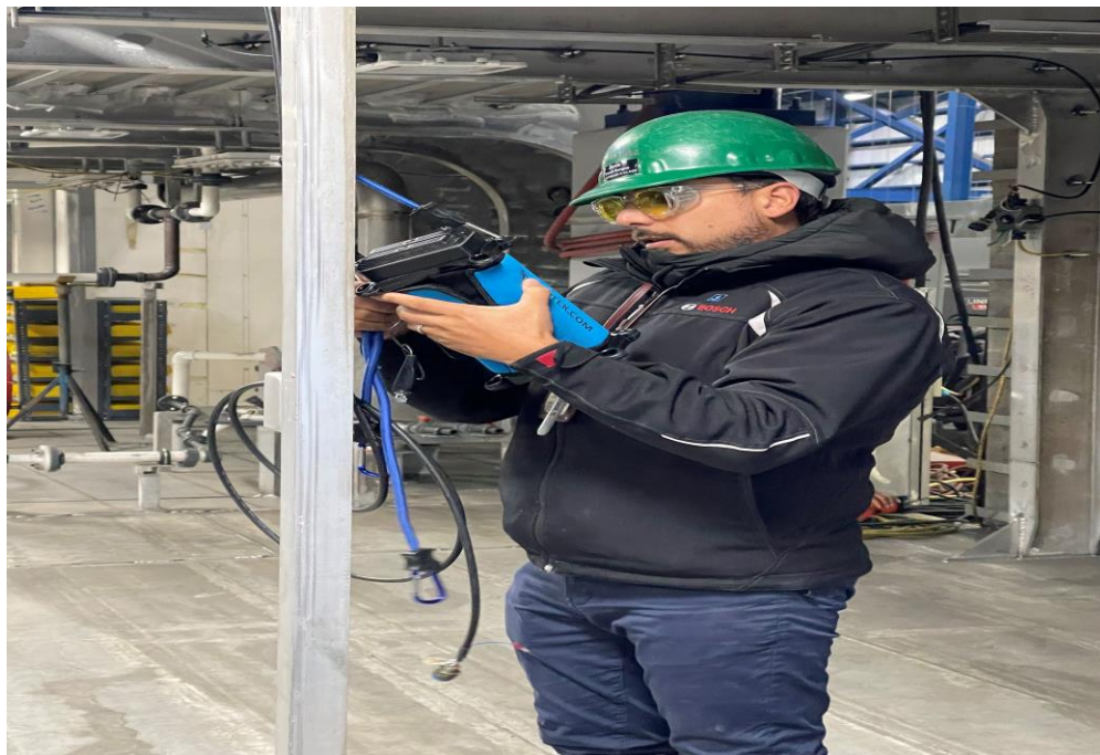
Figure 15. The same technician just completed wire termination of a cable can then proceed with the quality control acceptance testing using the AMUET TBU300SAP and AMUET TBU150HV testers to confirm continuity, DC resistance values and high voltage insulation resistance. Seen here is the technician installing an AMUET testers with bungee cable to reduce the stress on the cable installation.
