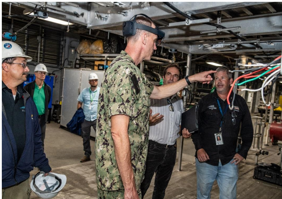
Figure 3. The US Navy was also very well-represented during RAP Final Demonstrations with SUPSHIP and NAVSEA04. Seen here is Rear Admiral Scott Brown wearing the HoloLens 2 to visualize working instructions for the cable routing of the AIDT demonstrator.
