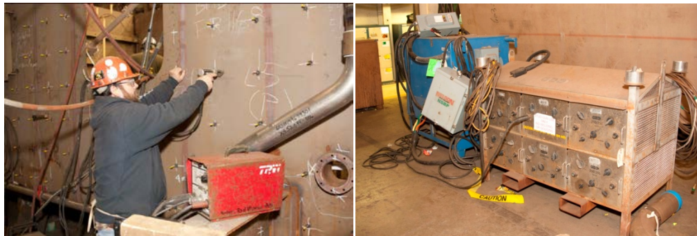
Figure 16. Pinning at BIW with timer box (left) and grid load and energy monitor (right)
