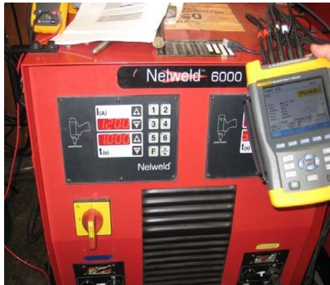
Figure 18. N800i with the Fluke Power Analyzer
