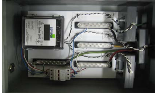
Figure 4. Energy meter enclosure shown here with a pigtail cord
