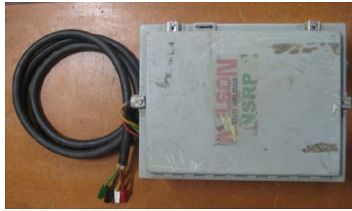
Figure 3. Inside view showing meter and CTs
