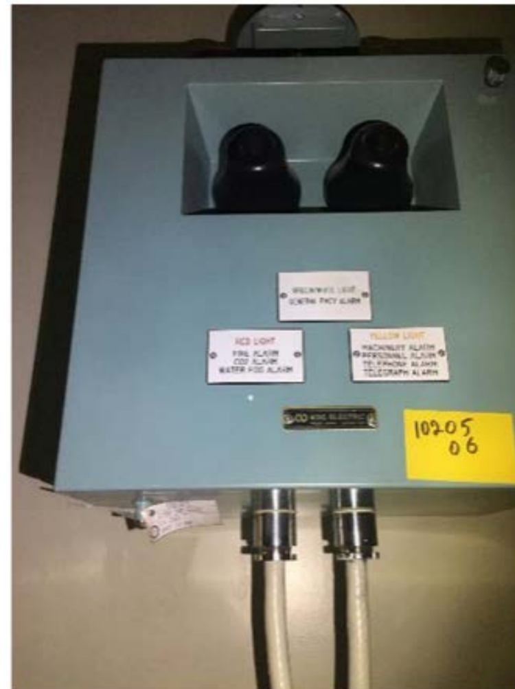
PC76 : Ensure Alarm Column in grounded
