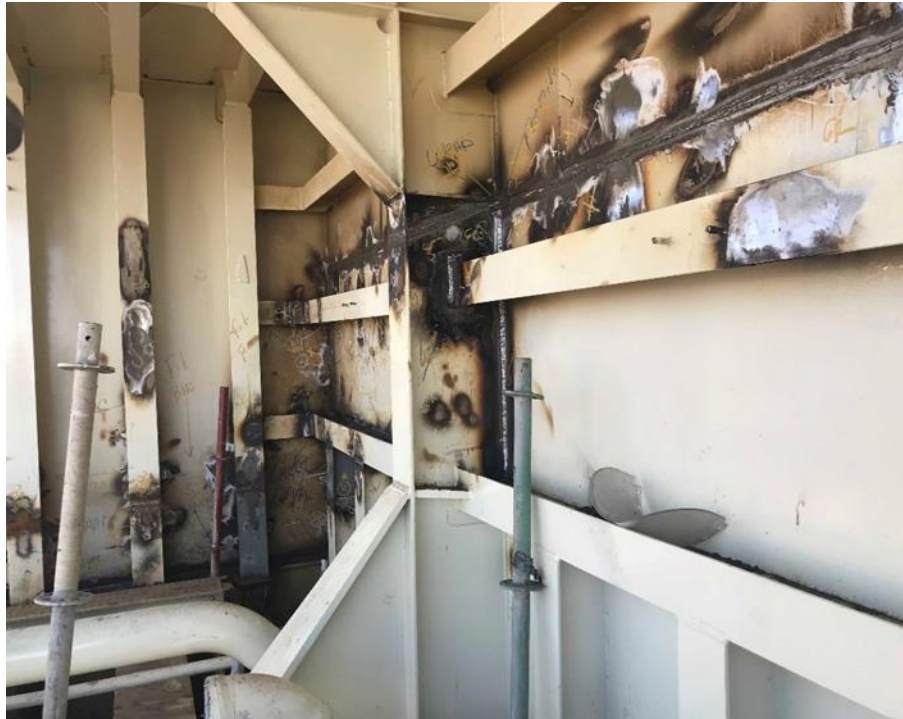
Figure 3. Hot Work Damage to Type VII (UHS) Epoxy.
