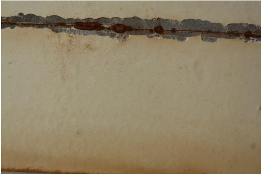
Figure 25. Least amount of Checking Displayed on Interbond 998
