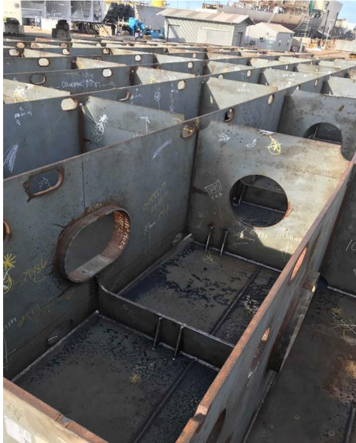
Figure 2. Degradation of PCP coated surfaces during unit construction.
