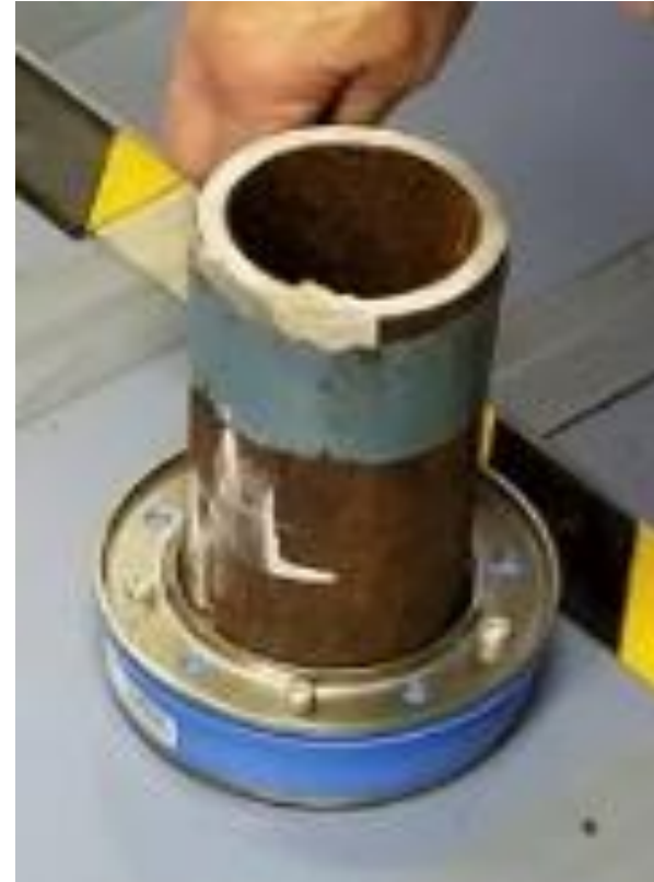
Tightening the SPM seal around the pipe before fixing the entire assembly to the bulkhead
