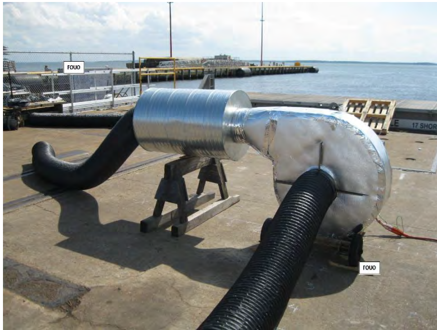
Figure 4 – Acoustical Jacket, as installed on the surface of the fan housing
