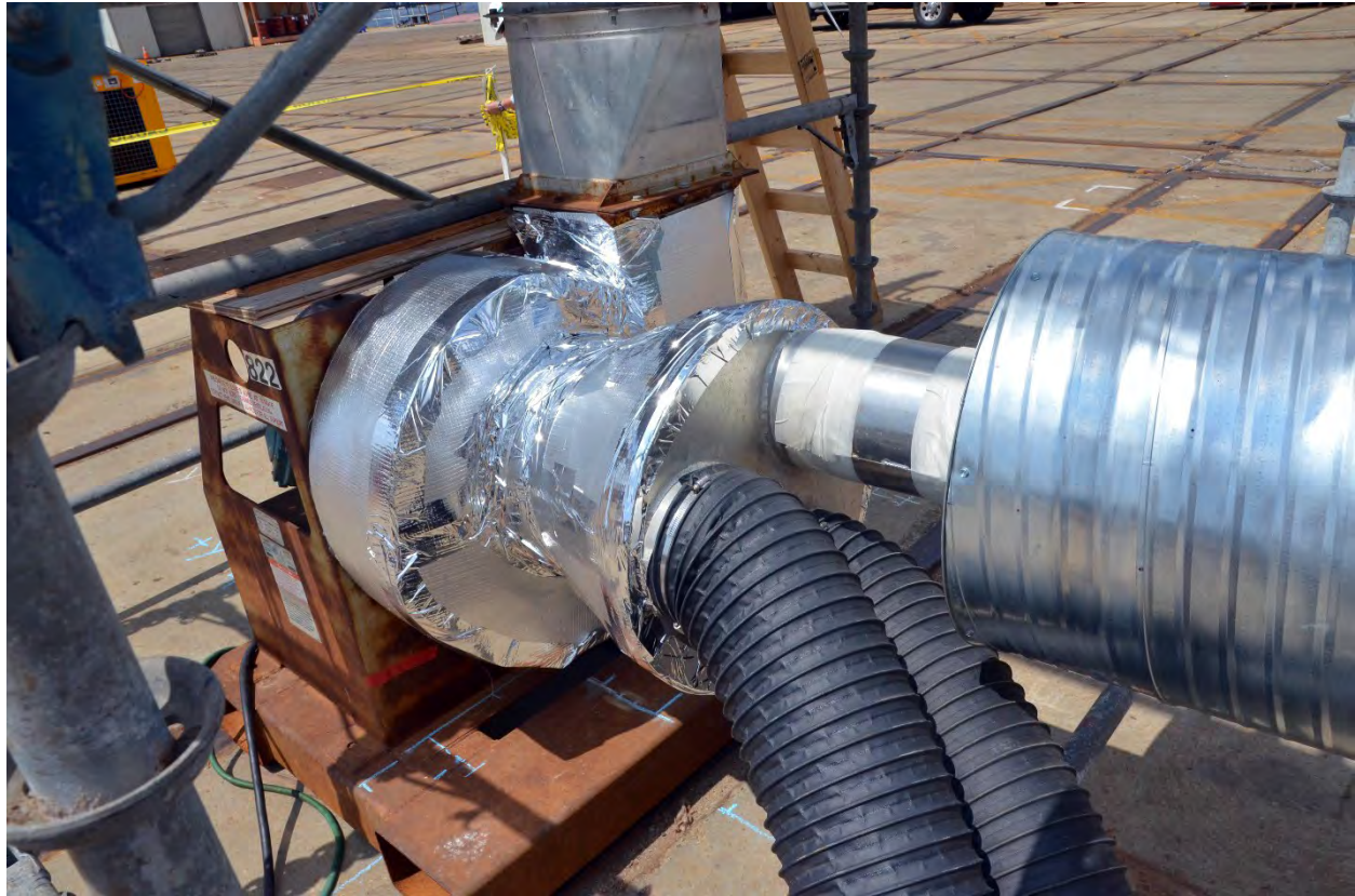
Figure 11 – Acoustical-jacket for Coppus TM-8, as tested
