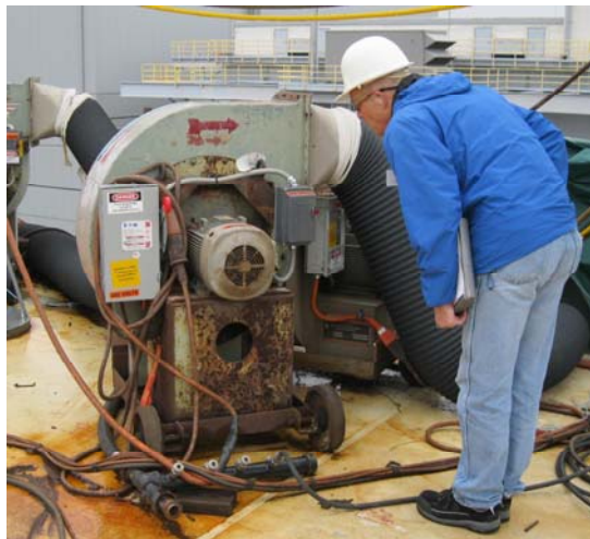
Figure 1 – Temporary Ventilation Blower
