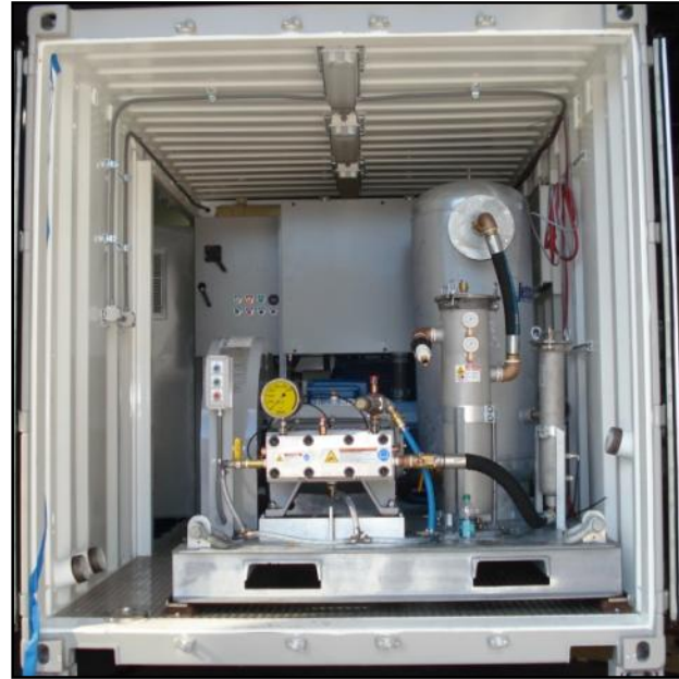
Electric UHP Pump in 20' Container
