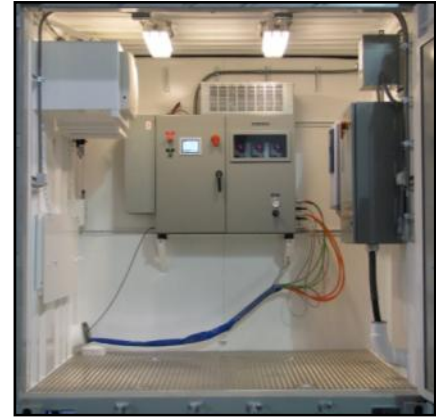
Example of Control Room
