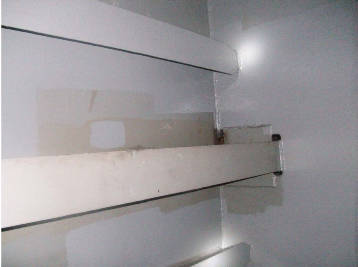
Figure 4. Stiffeners with retained PCP after 20 months in service.
