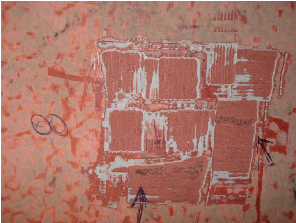
Mechanically exposed steel substrate at test location 8 – note two locations where corrosion is exposed.
