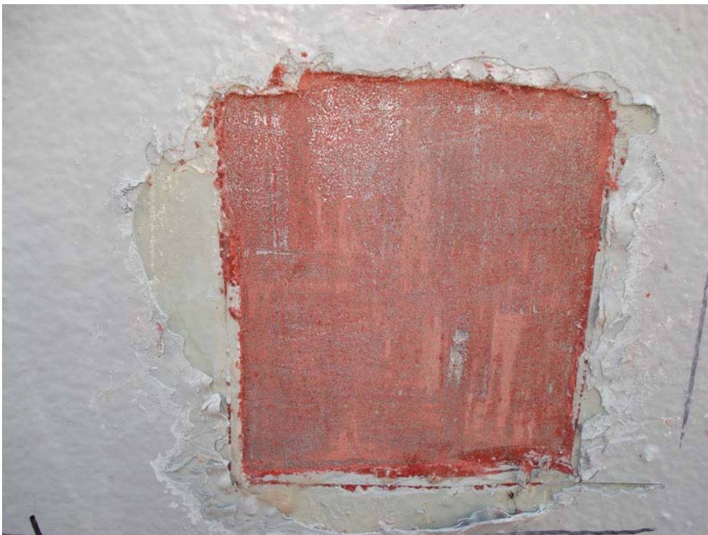
Exposed steel substrate at test location 2.
