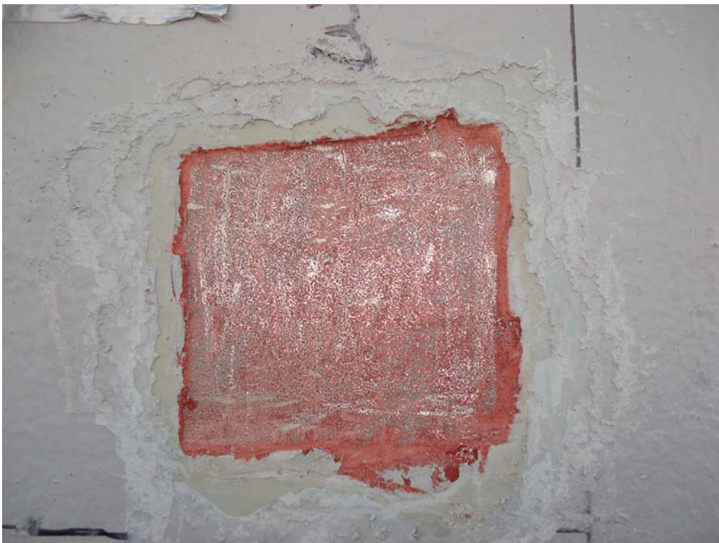
Exposed steel substrate at test location 3.
