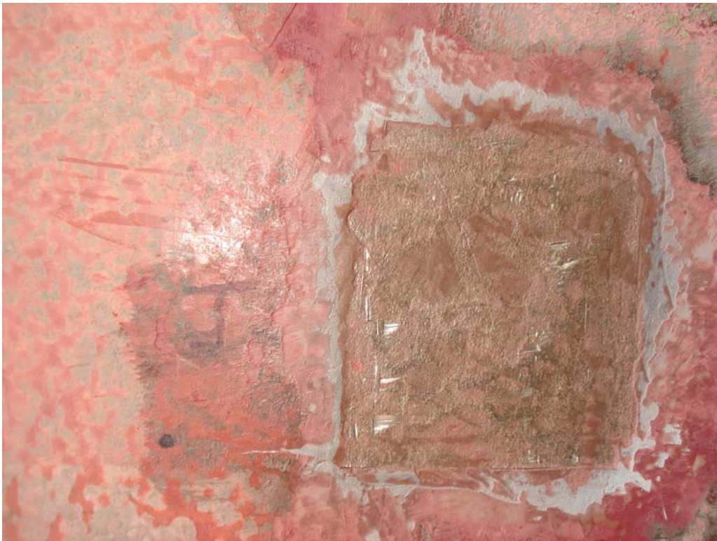
Exposed steel substrate at test location 4.
