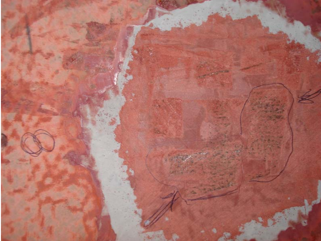
Exposed steel substrate at test location 8.
