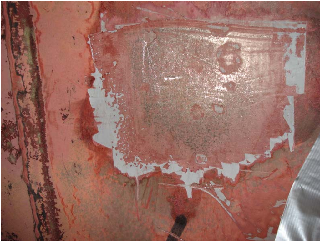
Exposed steel substrate at test location 1.
