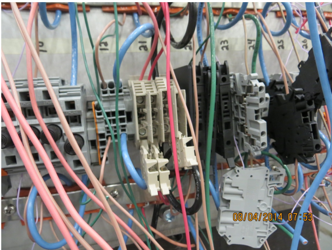
Photo 36 – File No. JP14-0175 View showing connector #21 disconnected and #22 partially disconnected from DIN rails
