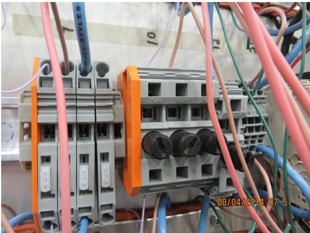
Photo 34 – File No. JP14-0173 View showing connector #10 disconnected from DIN rails after Shock Blow No. 3
