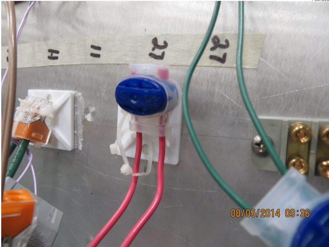
Photo 49 – File No. TE14-0582 View showing connector #27 with broken zip tie
