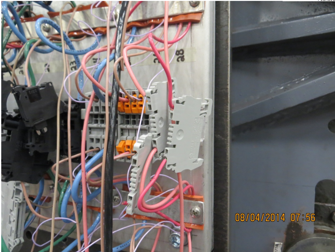
Photo 39 – File No. JP14-0178 View showing connector #28 disconnected from DIN rails after Shock Blow No. 3
