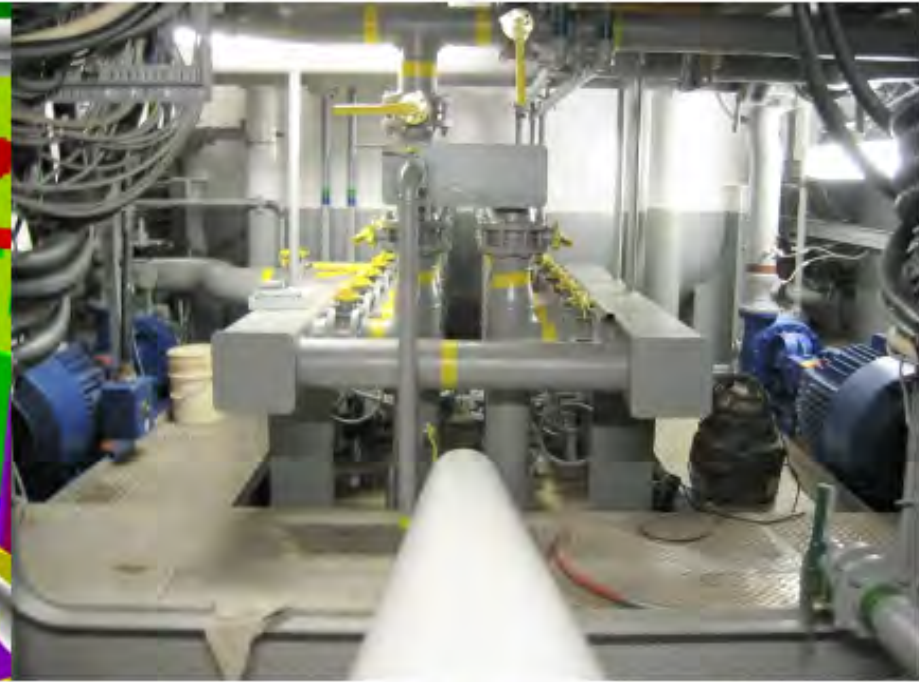
Picture of the actual Cargo Fuel Oil Manifold.
