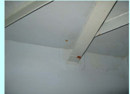
Ballast Tank after one year.
