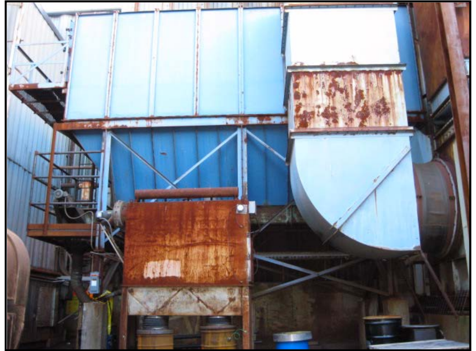
Abrasive blasting dust collectors
