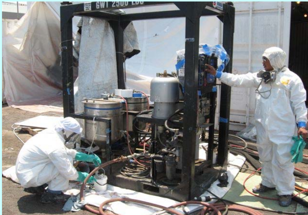
Custom GRACO 68 to 1 Extreme Mix Heated Plural Component Application Spray Pump Rig used to install June 2008
