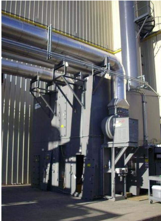
↑ VOC Abatement Equipment (Qty. 5)
